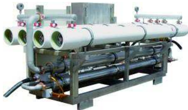
DCT 180t/day desalination plant.
